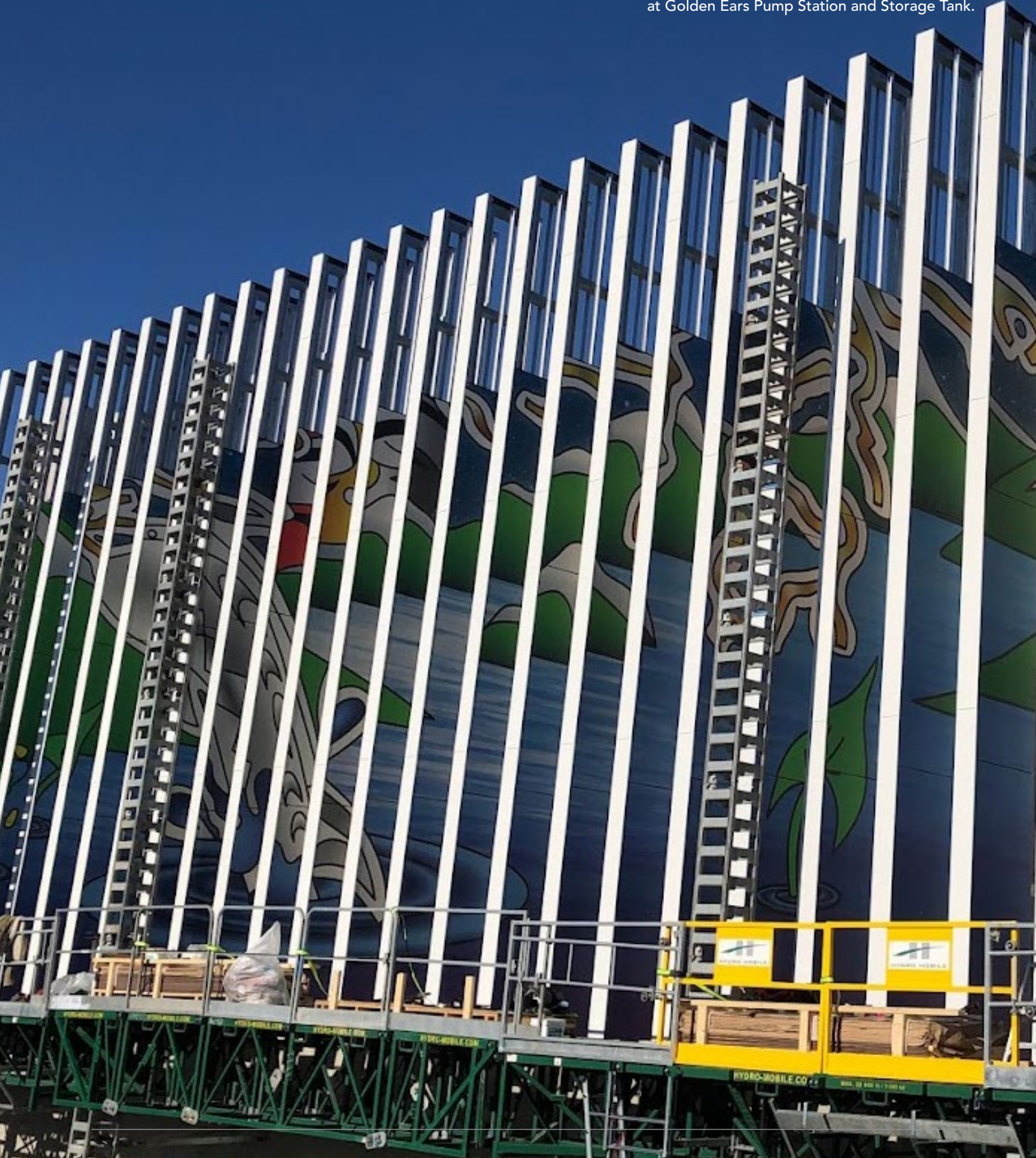
Installation of Katzie artist Rain Pierre's mural at Golden Ears Pump Station and Storage Tank.
